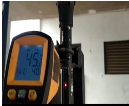
Figure 2 Flare temperature measurement using a thermometer
